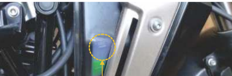
Coolant Expansion Tank
